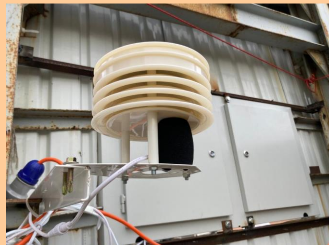
Sensor installed near by ASR/NSR
